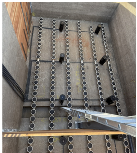
Large Bubble Mixers and Temporary Anaerobic (ANA) Basins
