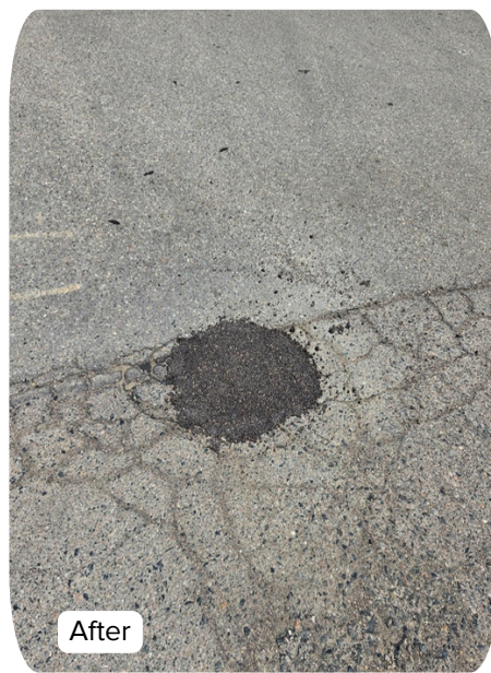
Potholes were filled around town.
