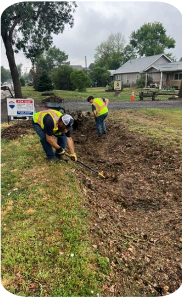
1st Street- Street crew cleaning up debris from the previous night's hailstorm
