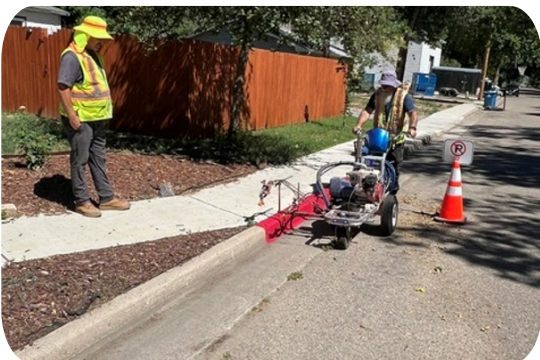
Welch & 7th Street- Streets crew continued identifying intersections where vehicles parked too close to corners, which created visibility concerns. Parking restrictions were implemented at Welch Avenue & 7th Street to improve sight distance and enhance safety for both drivers and pedestrians
