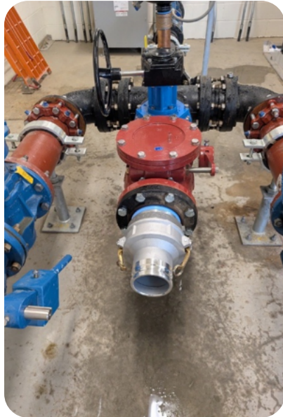
Heron Lakes Lift Station Emergency Bypass Valving
