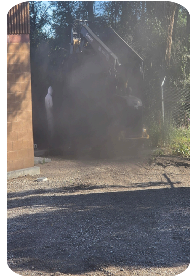
Water plant- Streets crew assisted the water plant each week by adding powdered activated carbon (PAC) to the water treatment system
