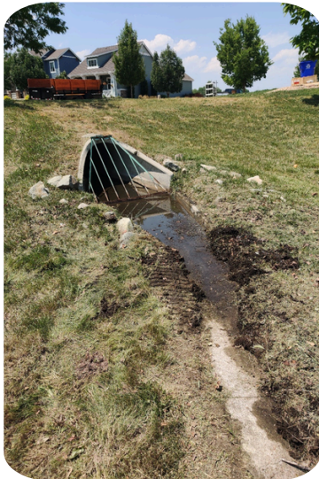
Collins Park- Streets crew cleaned the storm drain pan and outlet structure
