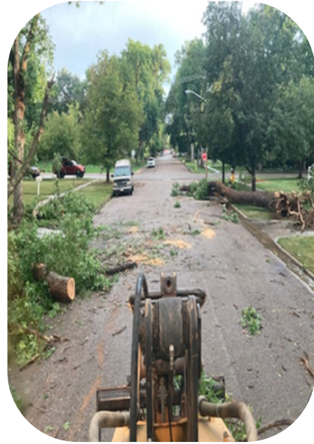
7th Street and Massachusetts- The streets crew was called in the help with downed trees from the recent storm
